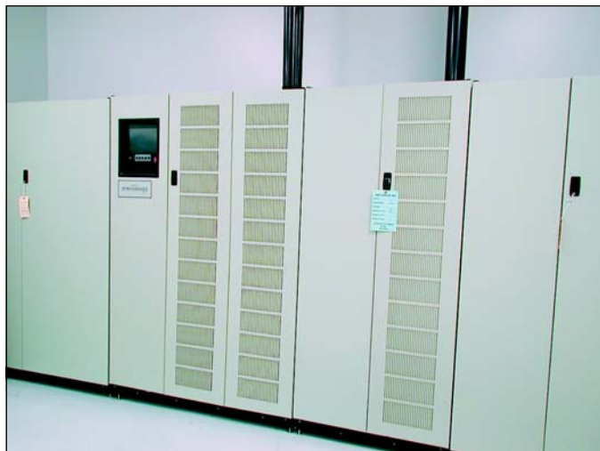
Figure 5. Redundant UPS units provide "clean," reliable power to the IDC.
