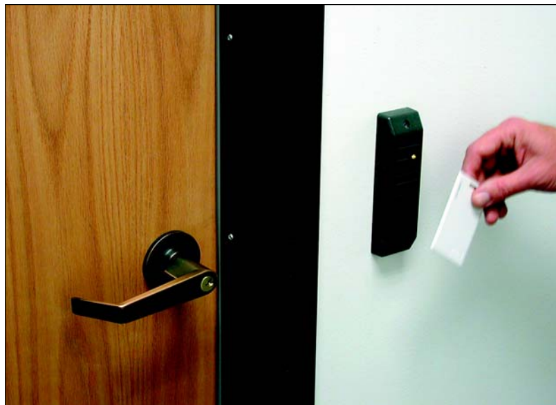
Figure 1. A programmable access card is used for high level IDC security.
