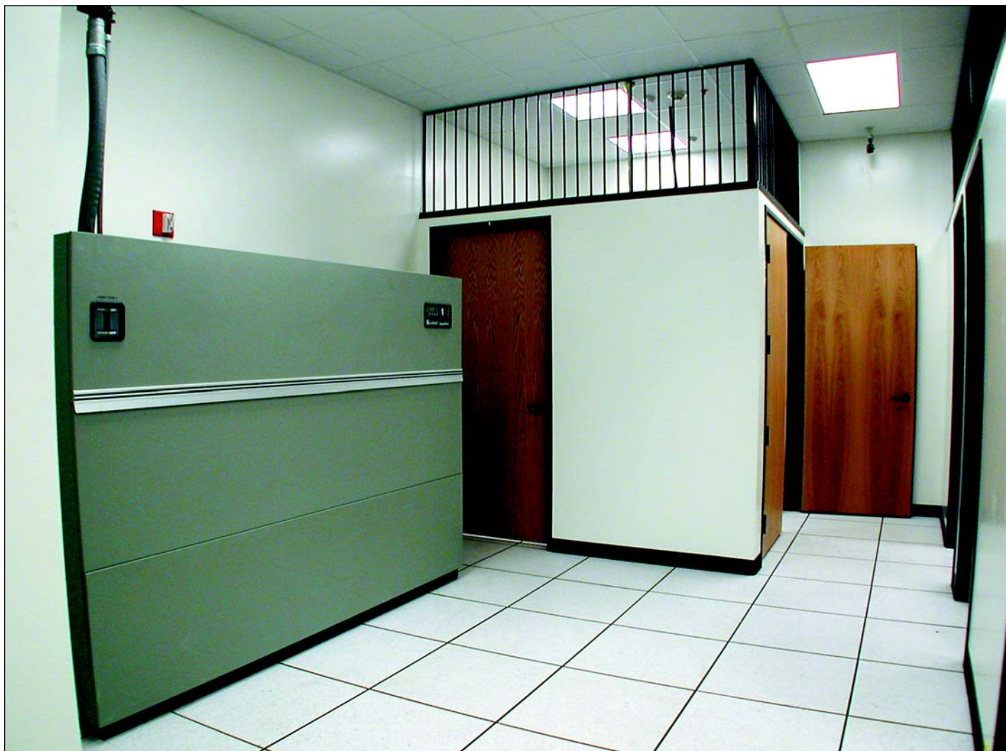
Figure 2. Temperature and humidity are maintained with redundant computer grade HVAC units.
