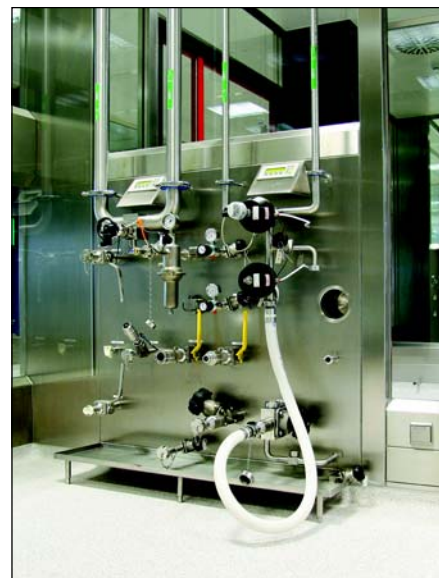
Flexible docking station for utilities and waste water.
